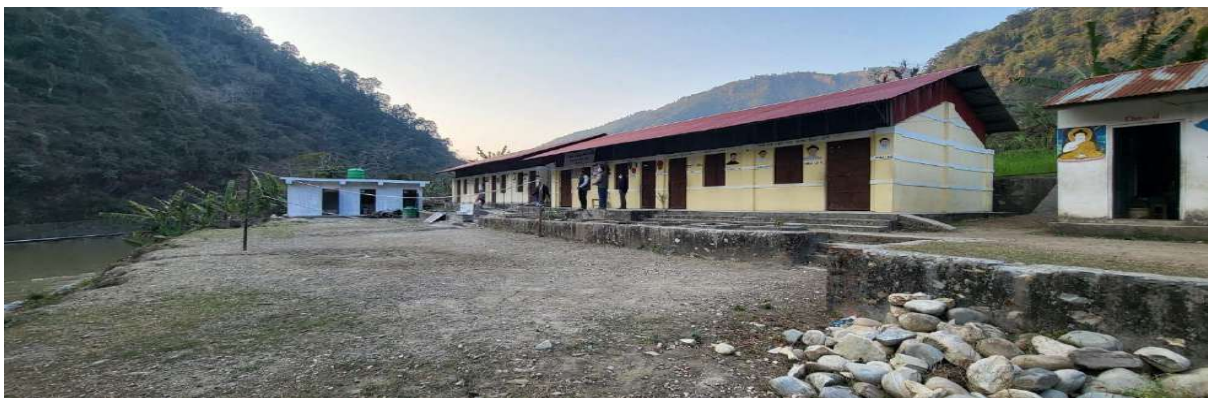
Figure 101: Affected School Building
